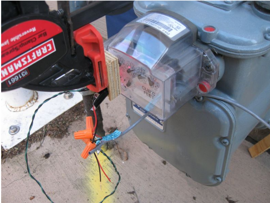
Contraption attached to gas meter. A red glow can be seen from the laser. The green/black wires go to the phototransistor.
