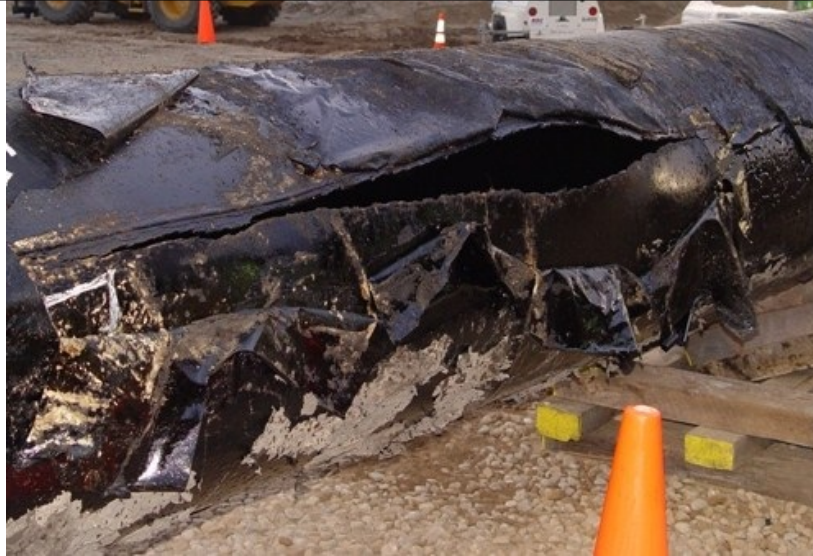
Enbridge's pipeline 6B, which ruptured July 26, in Michigan (Photo from NTSB)
