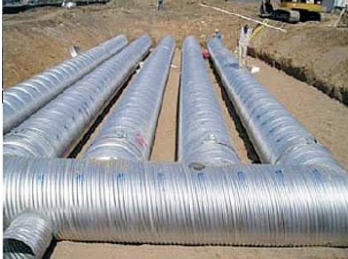
Drainage pipes on bentonite at the bottom of the test retort ( Red Leaf )
