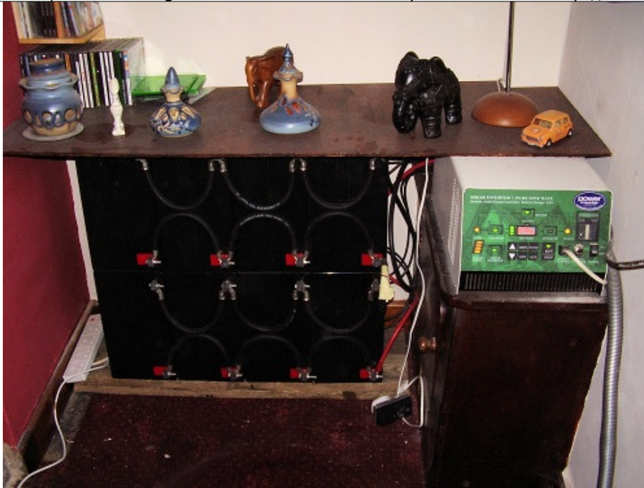
Batteries and inverter.
