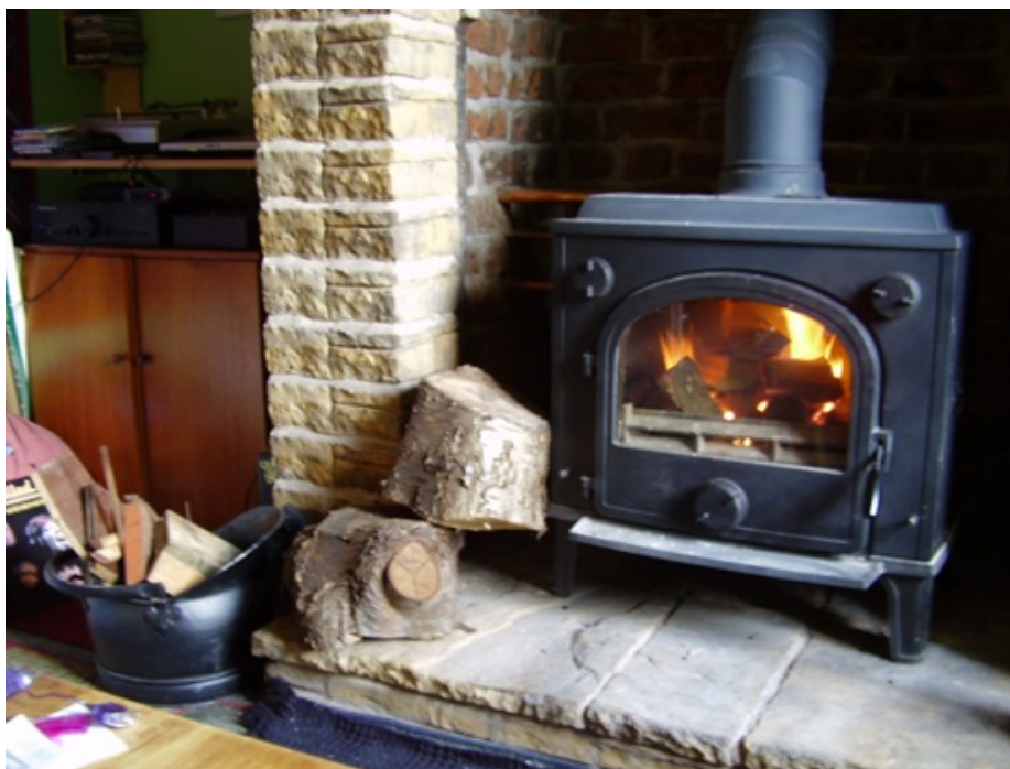
Wood burning stove with back boiler.
